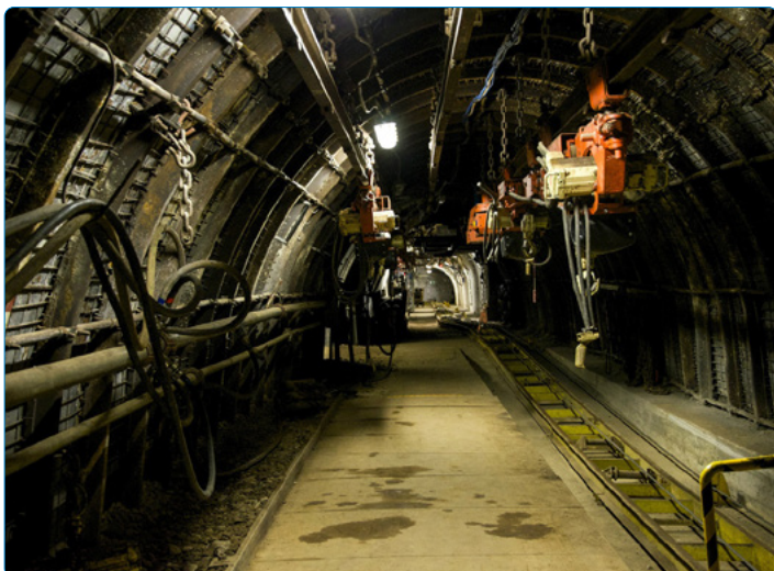
VHF TETRA improves coverage in dangerous underground locations, ensuring operations can continue and downtime is minimised.
